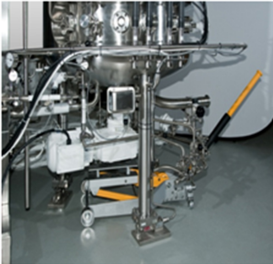
Gear box & Flowserve Double Mechanical seal
